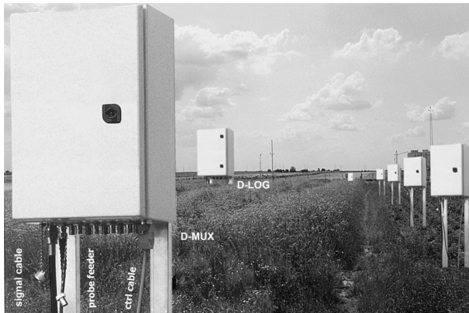
Fig. 20. An example of the D-LOG/10/mts-controlled stand incorporating six D-MUX/10/mts 2-nd level multiplexers. Maximum amount of the controlled FP/mts (or FP/m) probes is 60. For clarity only a single D-MUX was linked with the D-LOG and a single probe was connected to each D-MUX when taking the picture.
